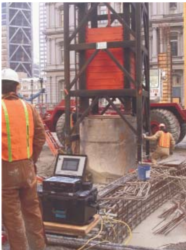
Figure 3. Dynamic load test of a drilled shaft using a 356 kN drop weight.
